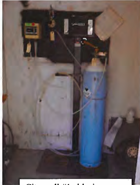
City well #1 chlorine gas
