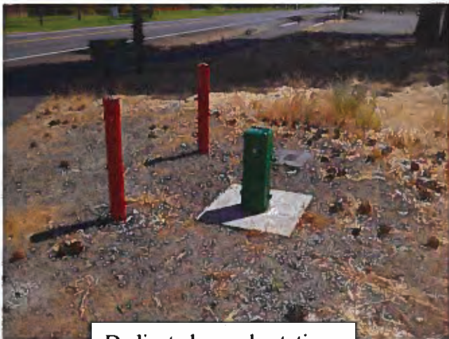
Dedicated sample station 1 of 3 in distribution
