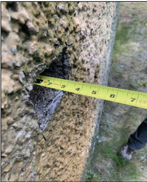
Figure 4: Exterior inspection window with no prestressing
