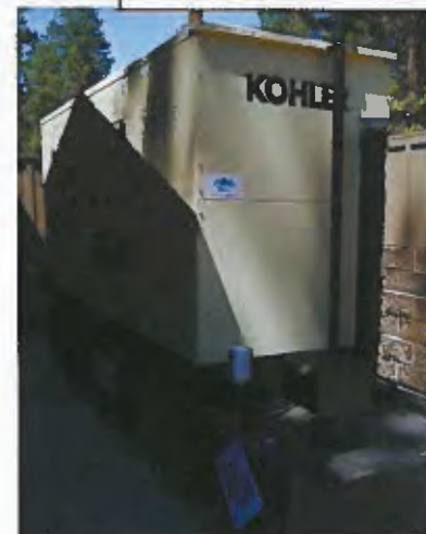
Back-up diesel generator for well #4
