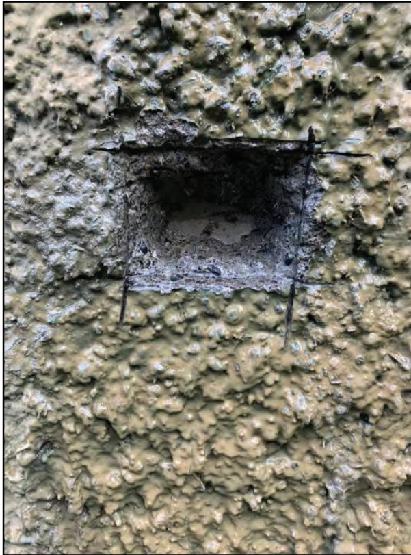
Figure 3: Exterior inspection window with no prestressing
