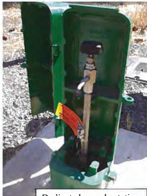
Dedicated sample station
