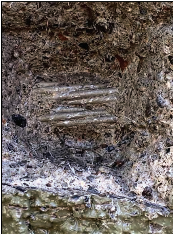
Figure 5: Exposed prestressing strand
