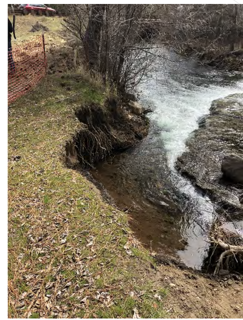
P3 BANK FAILURE ALONG NORTHERN FLOODPLAIN AT CONCRETE CAP
