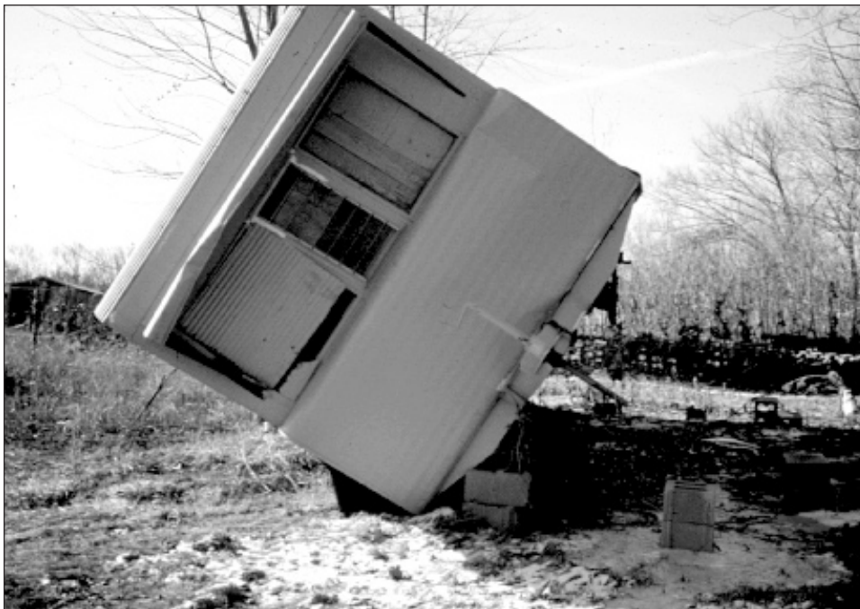
Figure 7-8. Failed foundation system that used masonry piers.
