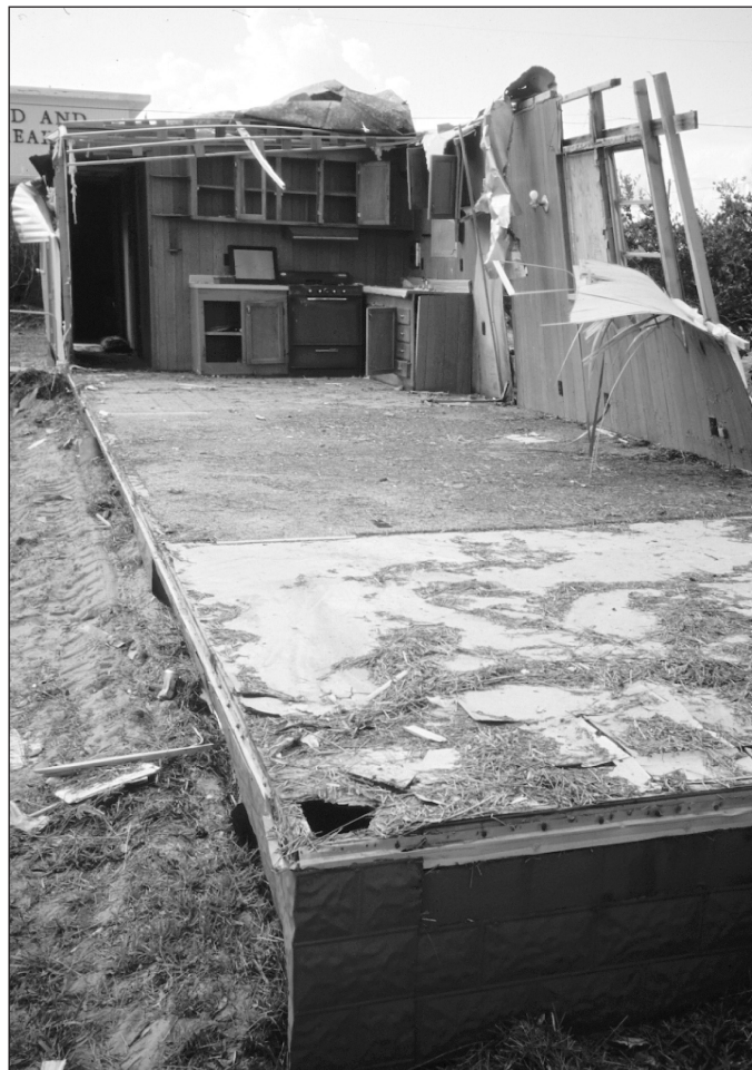
Figure 5-8. Failure of a modular home due to high winds. The home lifted off of its foundation (concrete slab) when the connections failed.
