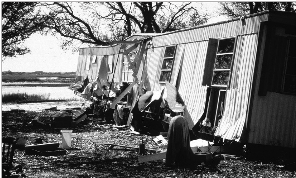
Figure 5-7. A manufactured home destroyed by the hydrodynamic forces of flooding.
