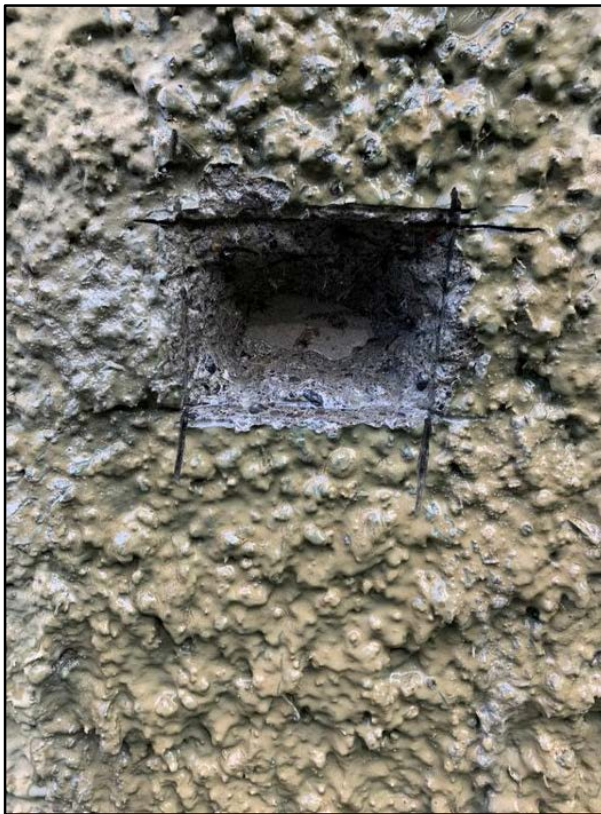
Figure 3: Exterior inspection window with no prestressing
