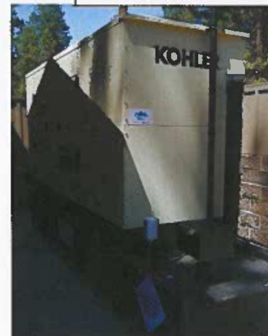
Back-up diesel generator for well #4
