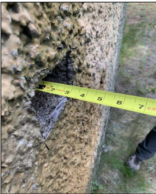
Figure 4: Exterior inspection window with no prestressing
