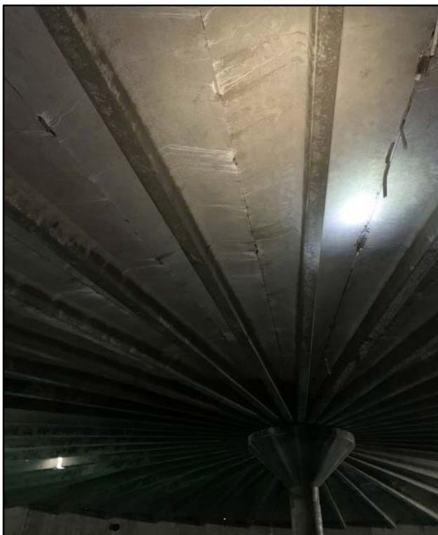
Figure 8: Interior view – note construction joints with existing spalls
