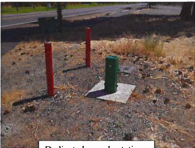
Dedicated sample station 1 of 3 in distribution
