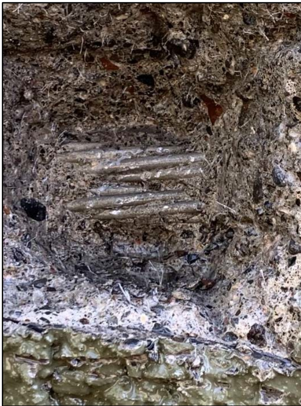
Figure 5: Exposed prestressing strand
