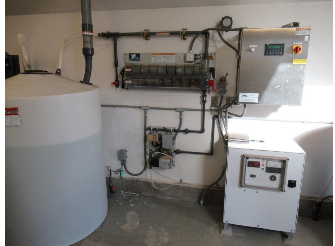
Onsite Hypochlorite Generation System
