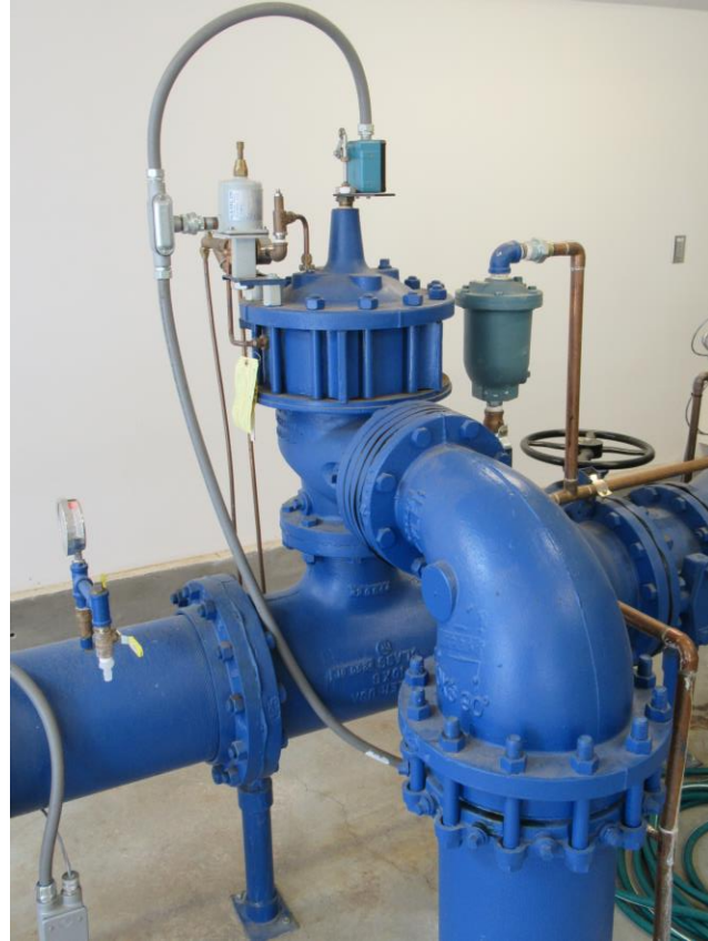
Deep Well Pump Control Valve
