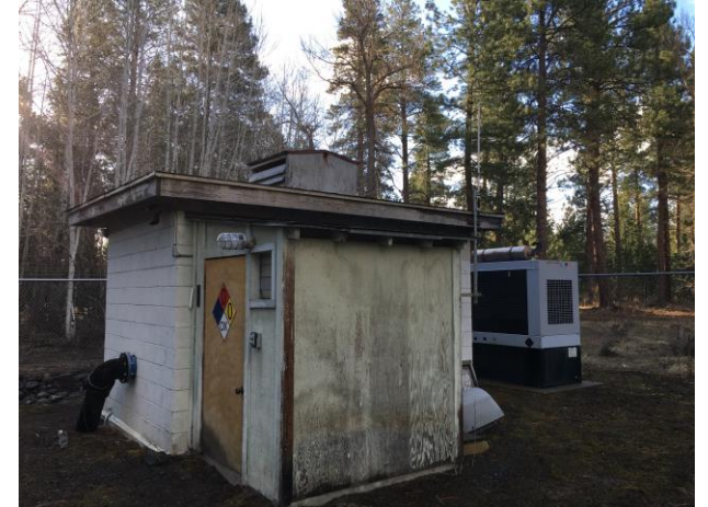
Existing Well No. 1 Pump Station
